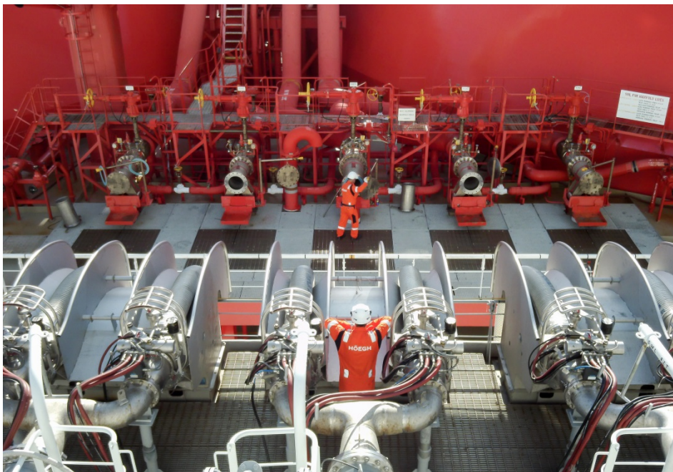
Figure 6 - ERS on FSRU manifold
