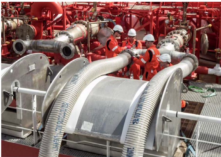
Figure 5 - Double hose support saddle on LNGC
